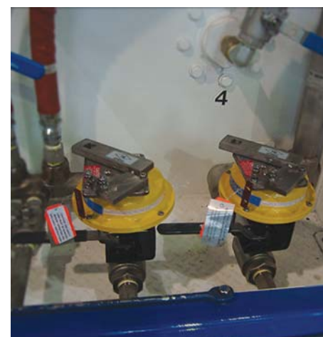
High pressure thermal shut-off assemblies for a compressed gas trailer.
