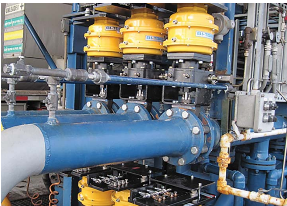
Bulk loading stations at a refinery.
