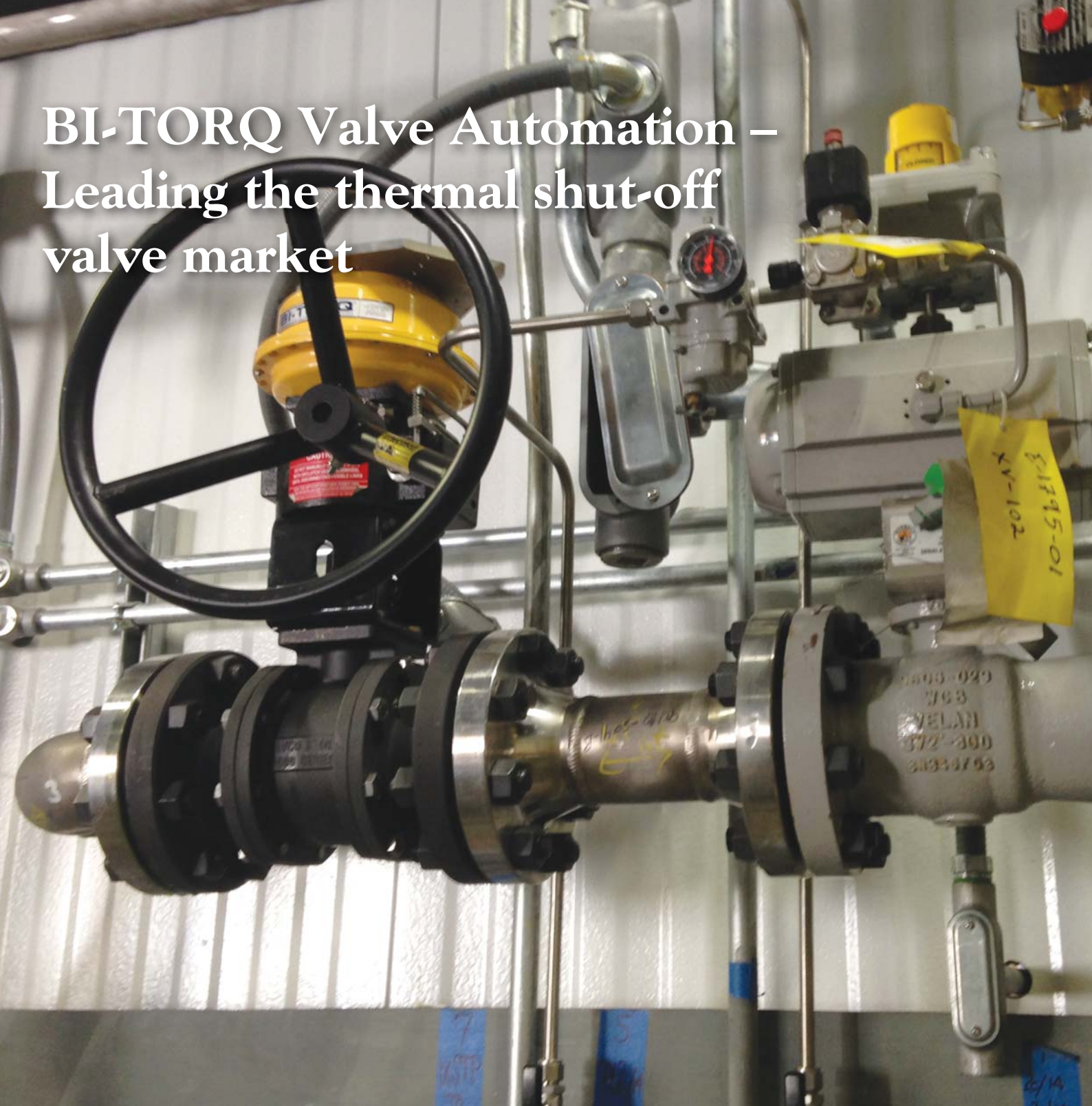
High pressure natural gas turbine installation.
